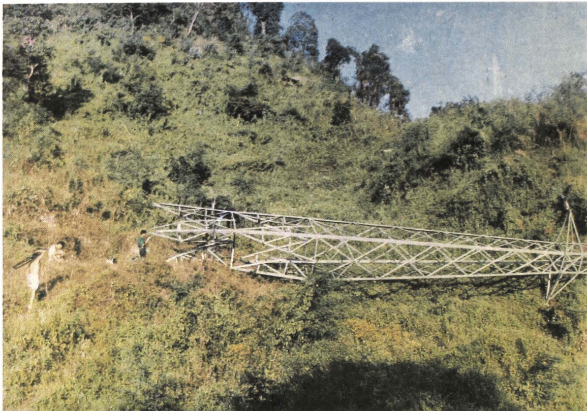
One of the several high tension electrical posts, supplying power to the Penden Cement Factory in Gomtu, felled by the anti-national terrorists.
