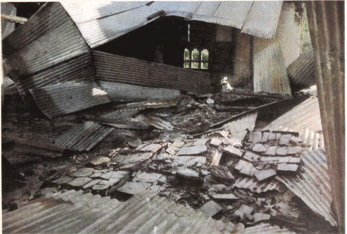
A section of a school in Samdrupjongkhar district destroyed by the anti-national terrorists.
