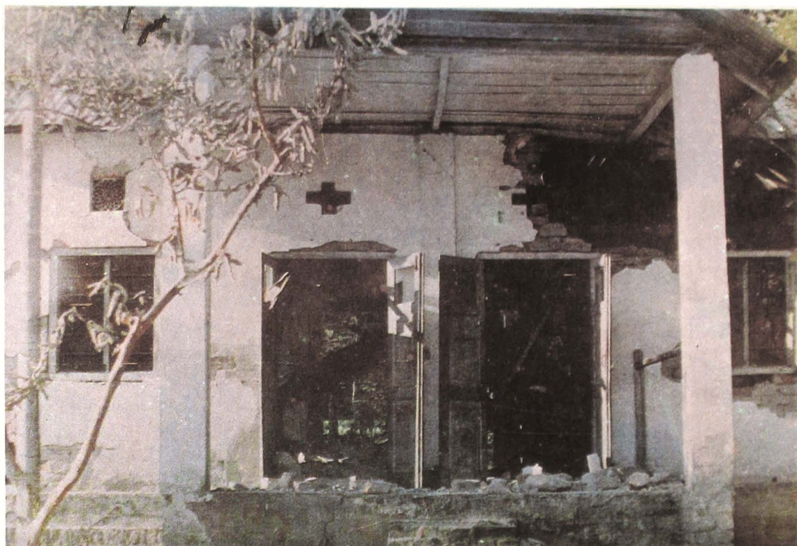
The Forest Beat Office at Daifam under Samdrupjongkhar District which was destroyed by the terrorists in early October 1990.
